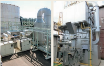
6 Combustion abatement system Striving to reduce emissions of environmentally harmful substances from the processes of producing specialty gas products and Ferro-chemicals.
