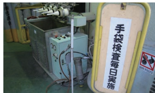
Glove inspection machine (made in-house) Small holes in the gloves used during operations can result in chemical burns. In order to prevent this, glove inspections are carried out prior to operations.
